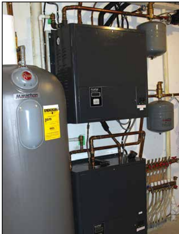
The heat pump water heater units that sit indoors and the tubing that circulates warm water to heat garage floors to entire homes. This new system offers efficiencies up to 300 percent.
