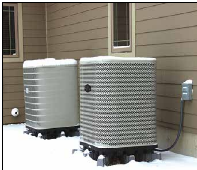
One air source heat pump water heater unit heats the lower level floor and one heats the garage floor.
