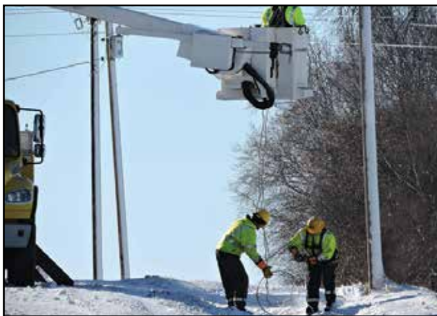
Line crews from MCPA and Wright-Hennepin Cooperative Electric work to untangle conductors and get lines back up south of Hector on November 19.
