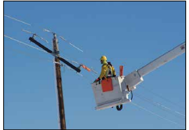
Lineman Kevin LaCourse works to repair cross arms on a pole north of Hector. Lineman worked two days in cold, strong winds to get power restored to all members.
