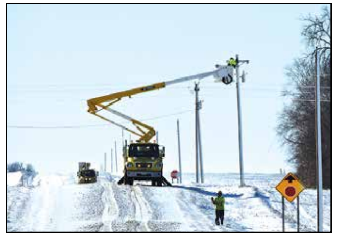
MCPA called in mutual aid crews from Hutchinson Utilities, Glencoe Light and Power, Wright-Hennepin Cooperative Electric, and Highline Construction to get all members back on before Saturday night. Due to the large number of outages across more than 16 townships many members were in the dark Friday night, Nov. 18. The Cooperative greatly appreciates the patience of our members who toughed it out through the storm.
